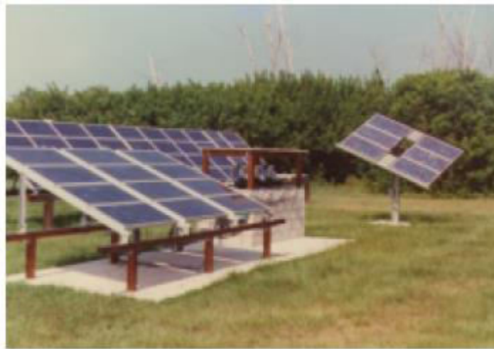
Rack and Pole mounted Arrays
